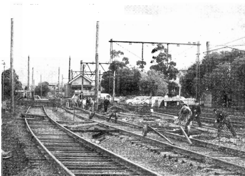
At left of picture are the temporary tracks at Napier Street, Footscray. These were being laid to permit work on the substructure to begin.
