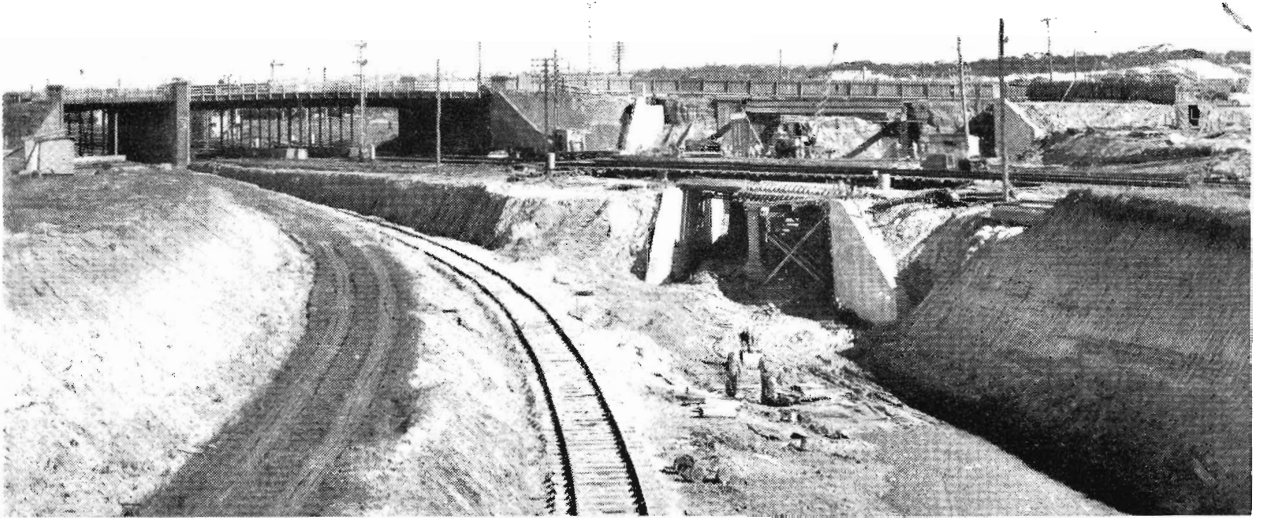
View from Bent Street, looking towards Princes Highway. The flyover bridge is in foreground and behind it is the new Princes Highway bridge. At left is the existing Princes Highway bridge. Track in foreground is that leading to grain elevators.
