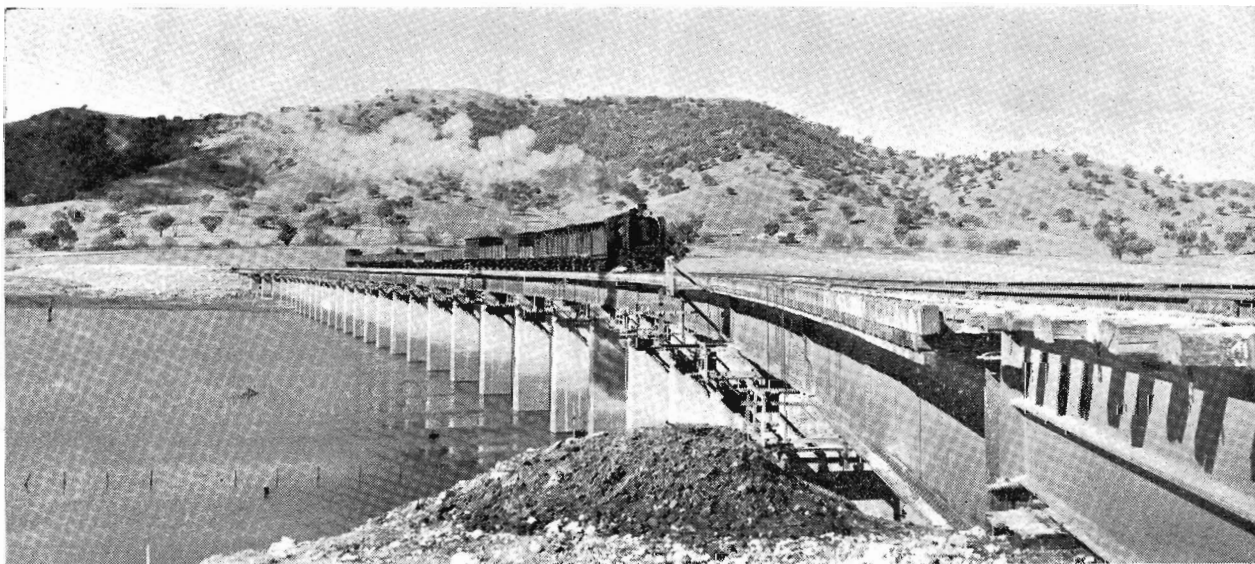
Sandy Creek bridge, partly raised and with the new spans at each end.
