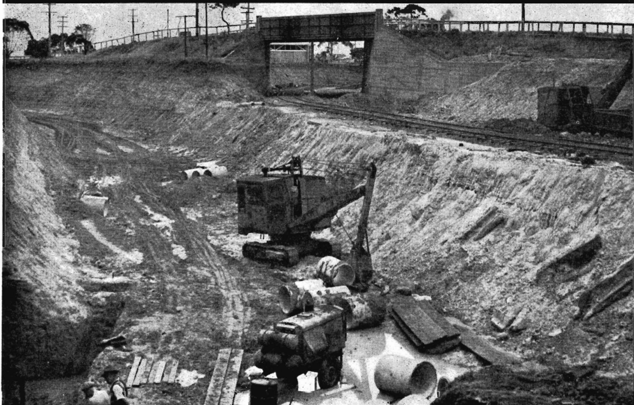
GEE LONG WORKS : Excavating for new tracks from new Corio Quay, which will pass under the main line near Separation Street. The project in the North Shore-North Geelong area involves the building of a flyover bridge to separate mainline traffic from that to the new Corio Quay, crossing under the Princes Highway, and lowering of tracks to the grain elevators. The completed work will permit handling of wheat, coal and other commodities without interference to mainline traffic.
