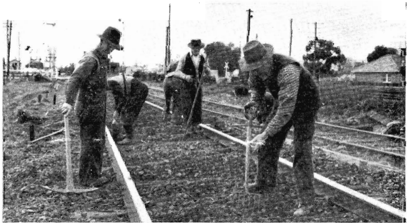
Ganger H. Wakenshaw and Repairers E. G. Watson, J. Findlay, R. Smith, A. E. Kneebone and F. Vyner re-sleeping track near station.
